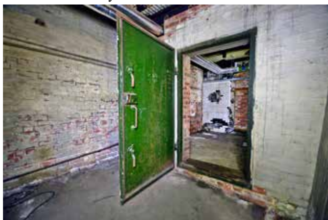
Heavy blast door at the entrance to one of the air-raid shelters
